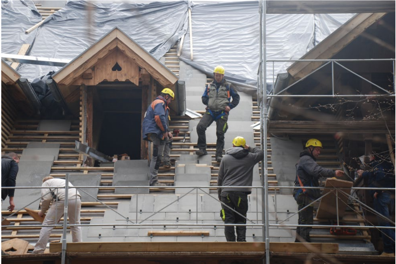
Roof covering with insulation in Ljubljana, Slovenia, 2016. Photographer: Tatjana Adamič © Institute for the Protection of Cultural Heritage of Slovenia, Tatjana Adamič
